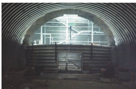
[1. Connecting an adit near the main tunnel with vertical shaft at 74 m dept]
