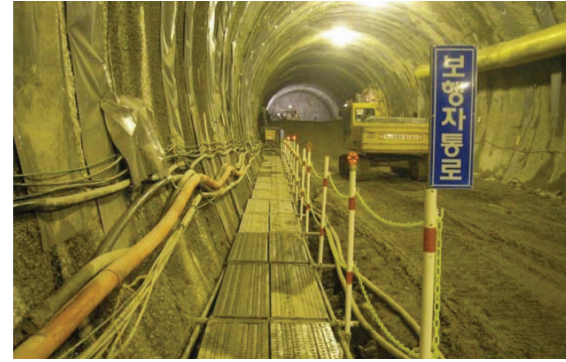
[Illumination management / Pedestrian passage to prevent collisions with vehicles]
